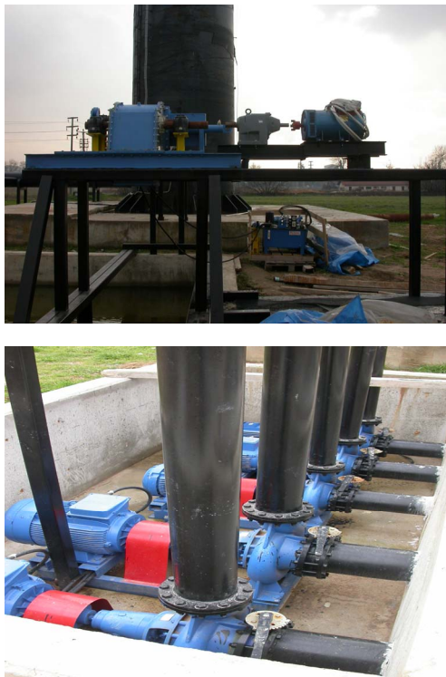
Fig.1. Pictures of the small hydro power system (overview and pumps)
